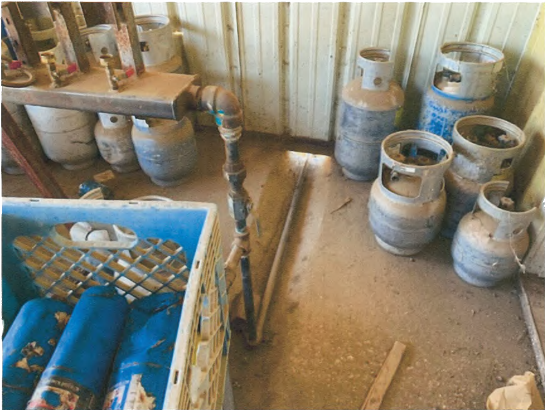
The two manifolds are hooked together and the line goes out to the vacuum tank.
