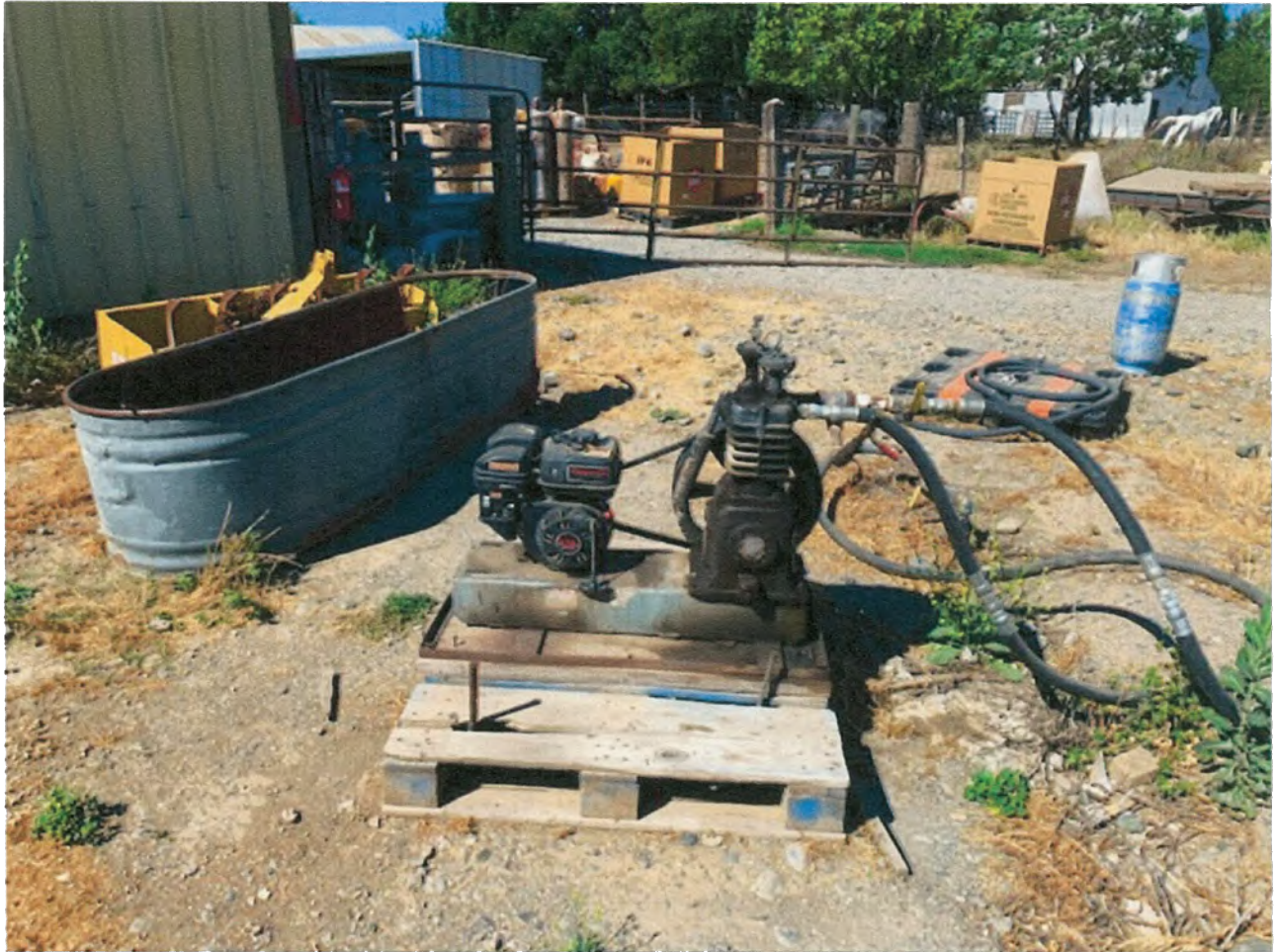
This is the vacuum pump. It takes the propane and stores it in the storage tank.
