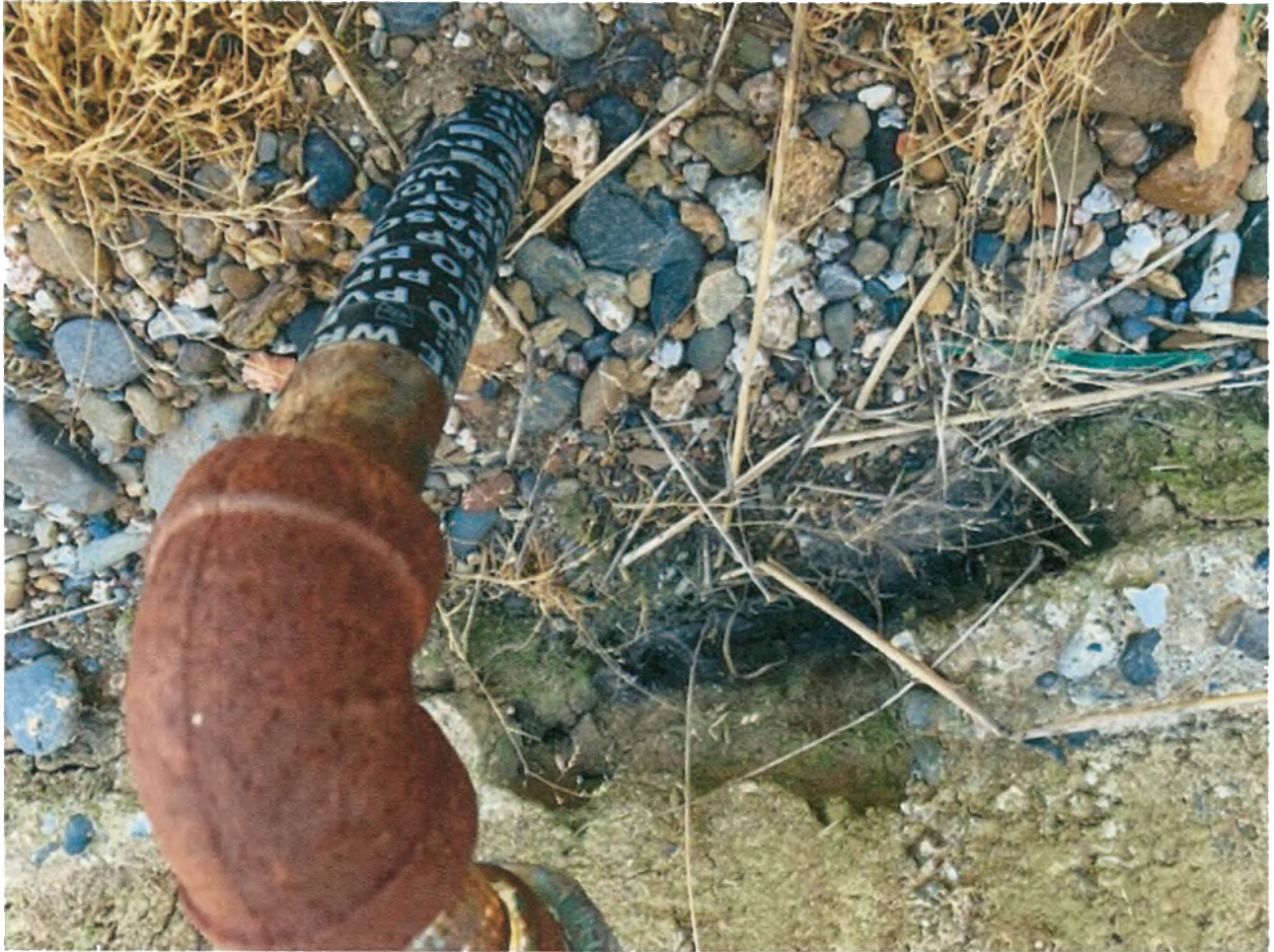
This shows the pipe being taped, the rest of the pipe under ground is taped as well.
